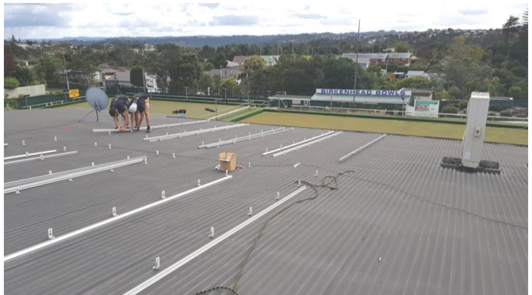
The beginnings of a good thing..... the installation of the solar panels have begun.
